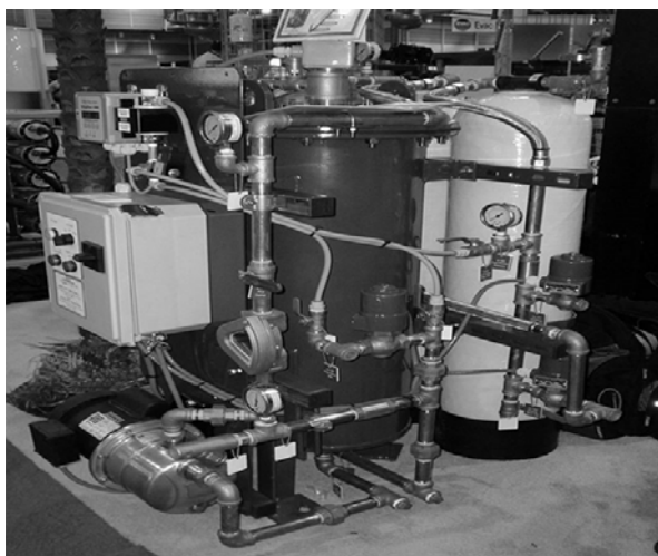
Figure 1. ship treatment / sewerage separator from machine area (marine oil water separator)
